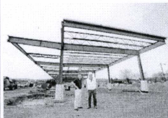
JAKE DANNA STEVENS / STAFF PHOTOGRAPHER COLTS Executive Director Robert Fiume, left, and construction manager Nicholas Custer on the site that will become the Lackawanna County intermodal transportation center in Scranton on Tuesday.
